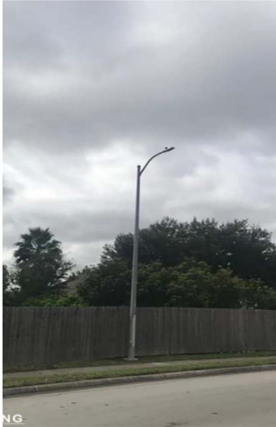
Existing CPS Energy Pole
