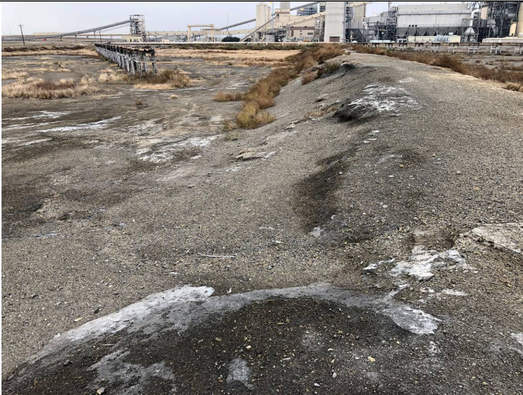
Photograph: 22 South Bottom Ash Pond – standing on northeast corner – facing west. Photo taken 12/15/2020.
