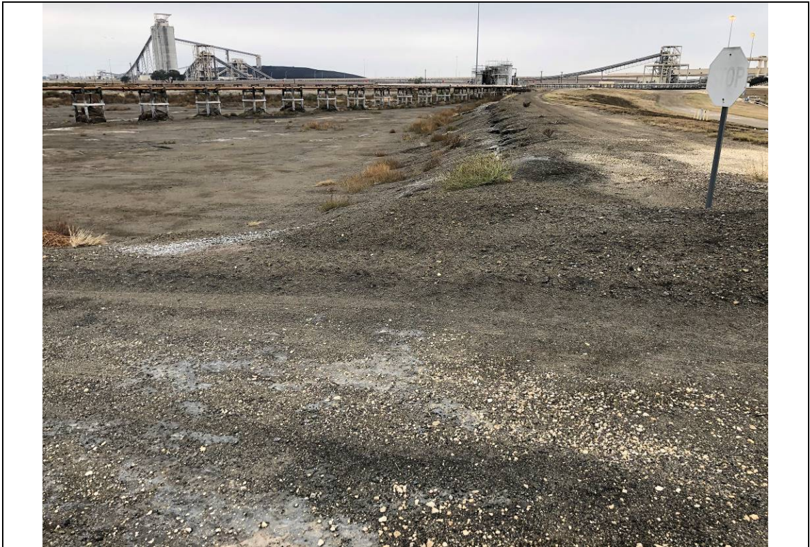
Photograph: 18 North Bottom Ash Pond – standing on northwest corner – facing southwest. Photo taken 12/15/2020.
