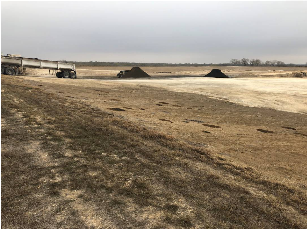
Photograph: 2 Fly Ash Landfill – standing on west berm – facing northeast. Photo taken 12/15/2020.
