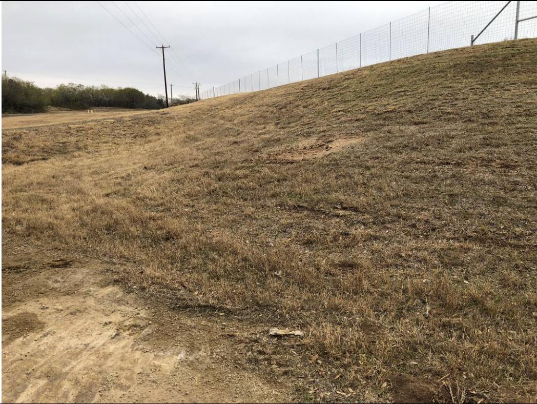
Photograph: 15 Evaporation Pond – standing on the southwest corner – facing north. Photo taken 12/15/2020.
