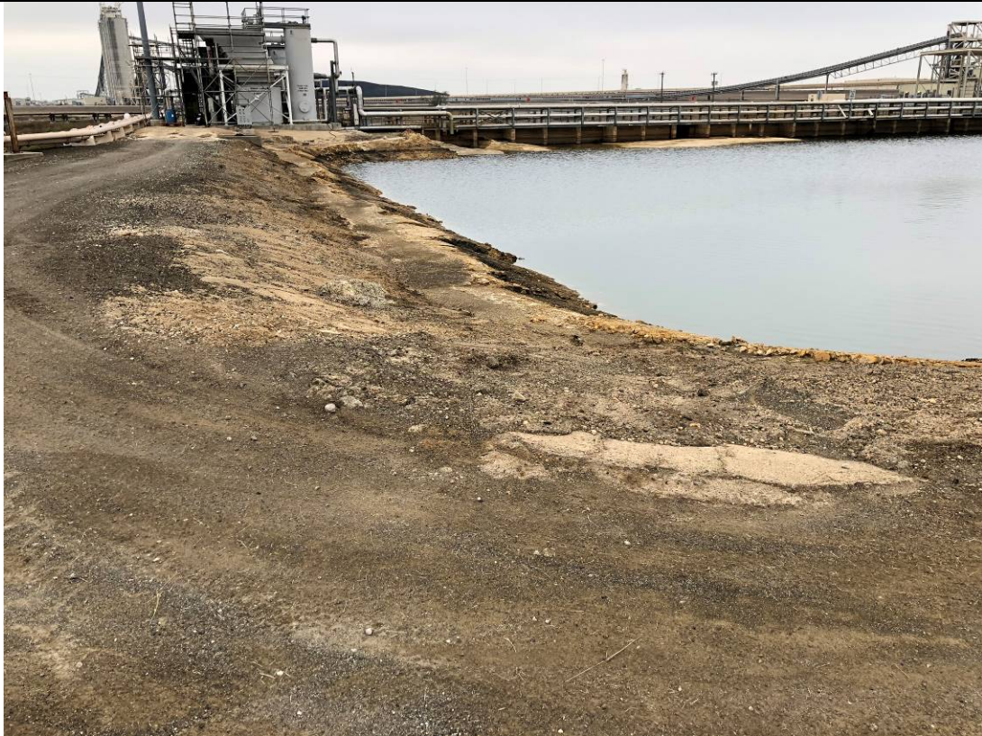
Photograph: 25 North SRH Pond – standing on northeast corner – facing south. Photo taken 12/15/2020.
