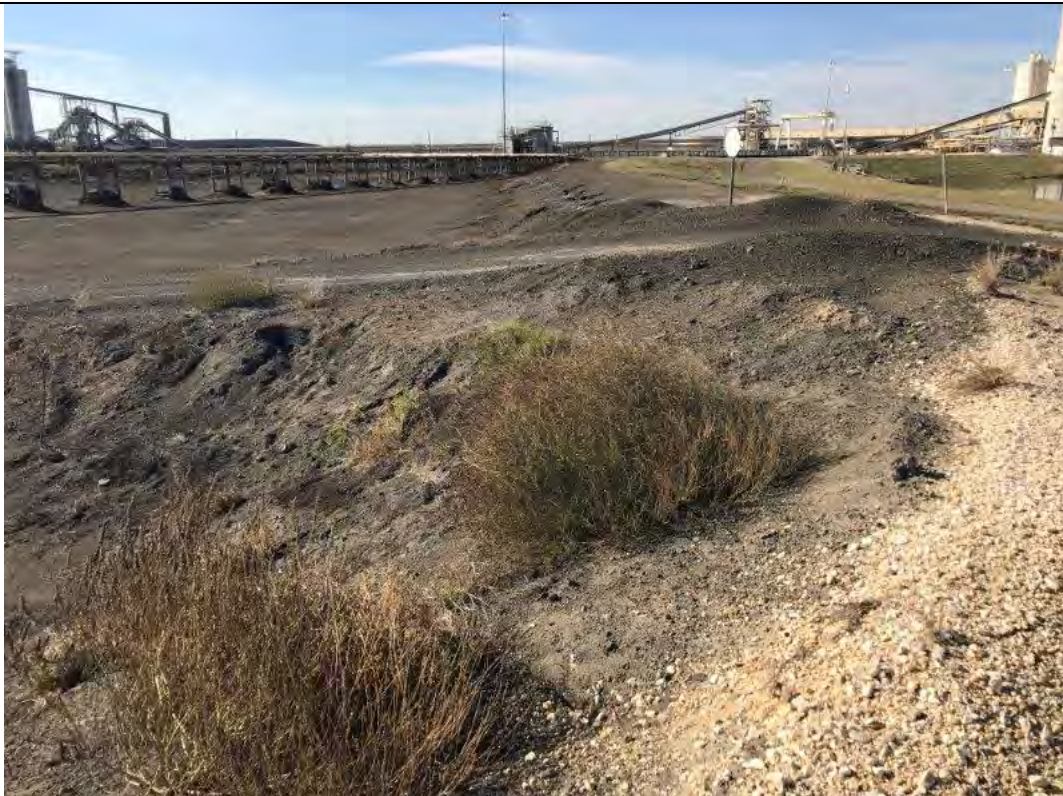
Photograph: 14 North Bottom Ash Pond – standing on northwest corner – facing southwest. Photo taken 12/19/2019.
