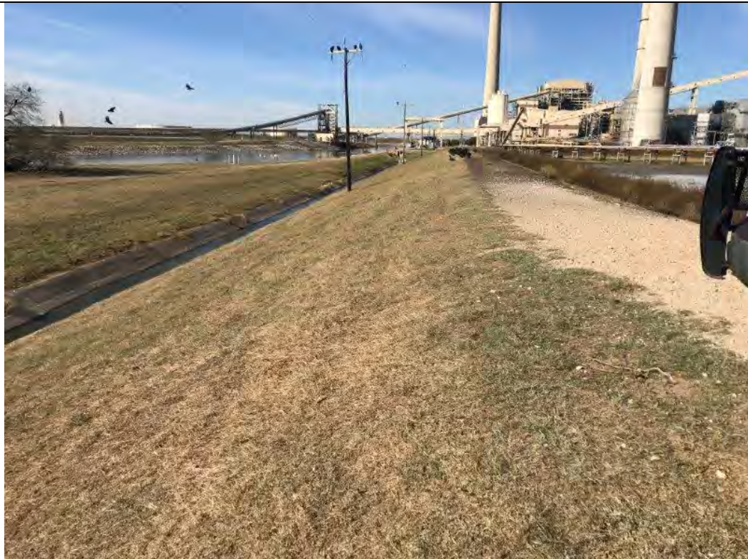
Photograph: 23 South Bottom Ash Pond – standing on southern berm – facing west. Photo taken 12/19/2019.
