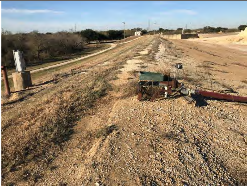
Photograph: 5 Fly Ash Landfill – standing on south berm – facing west. Radial stacker located in southwest corner and stormwater discharge piping in southeast corner of landfill. Photo taken 12/19/2019.
