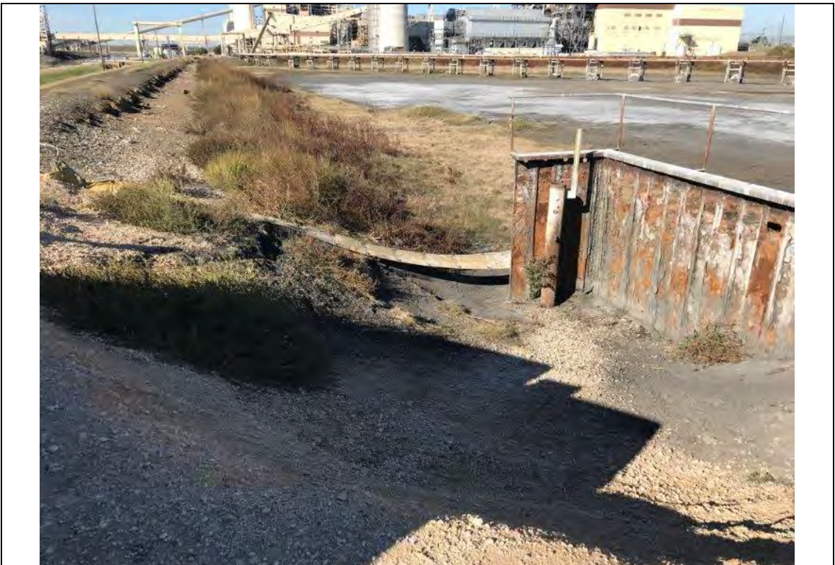
Photograph: 22 South Bottom Ash Pond – standing on southeast corner – facing west. Corrosion observed in vertical overflow pipe and sheet piling. Photo taken 12/19/2019.
