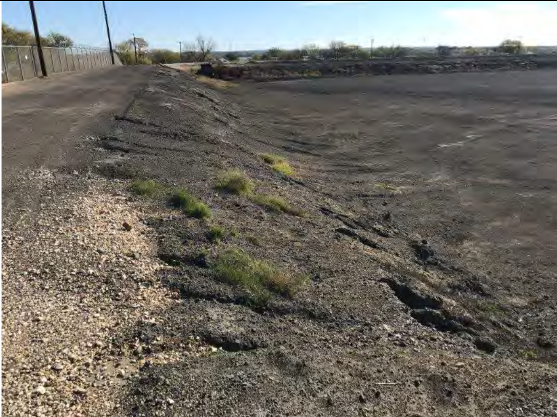
Photograph: 13 North Bottom Ash Pond – standing on northwest corner – facing east. Minor erosion observed on interior slopes. Photo taken 12/19/2019.
