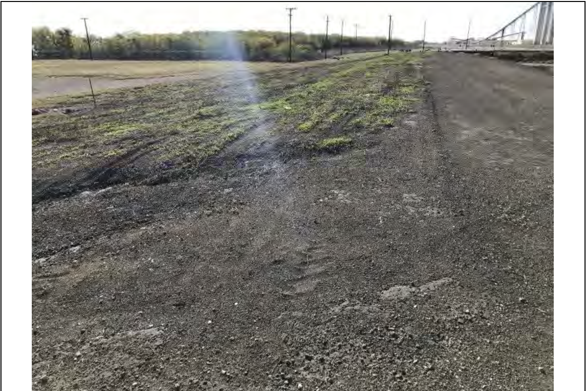
Photograph: 21 South Bottom Ash Pond – standing on eastern berm – facing south. Photo taken 12/19/2019.
