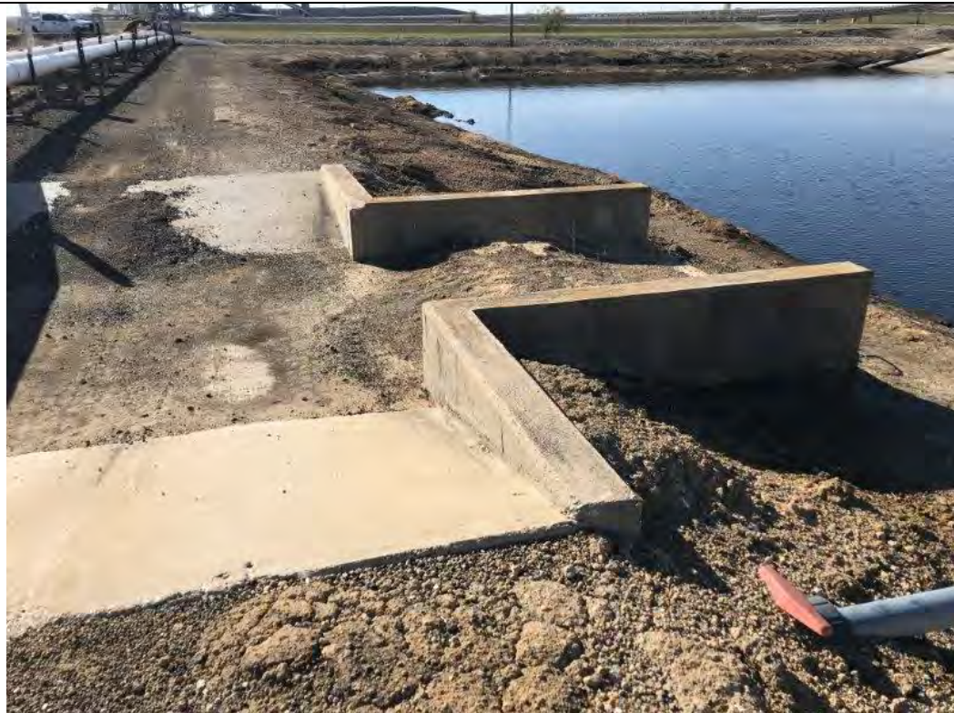
Photograph: 33 South SRH Pond – standing on the eastern berm – facing south. Spillway structure. Photo taken 12/19/2019.
