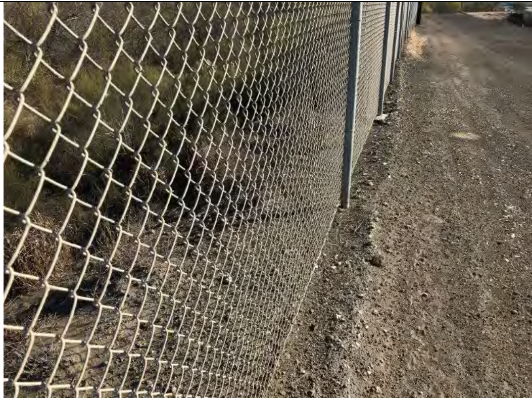
Photograph: 15 North Bottom Ash Pond – standing on north berm – facing east and down. Woody plant growth noted on north berm exterior side slope. Photo taken 12/19/2019.
