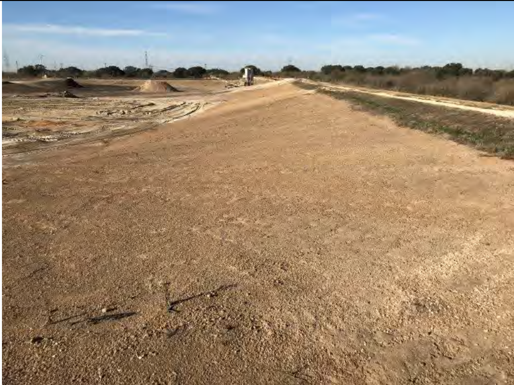
Photograph: 1 Fly Ash Landfill – standing on northern berm – facing west. Mobile ash conditioning machine located in northwest corner of landfill. Photo taken 12/19/2019.
