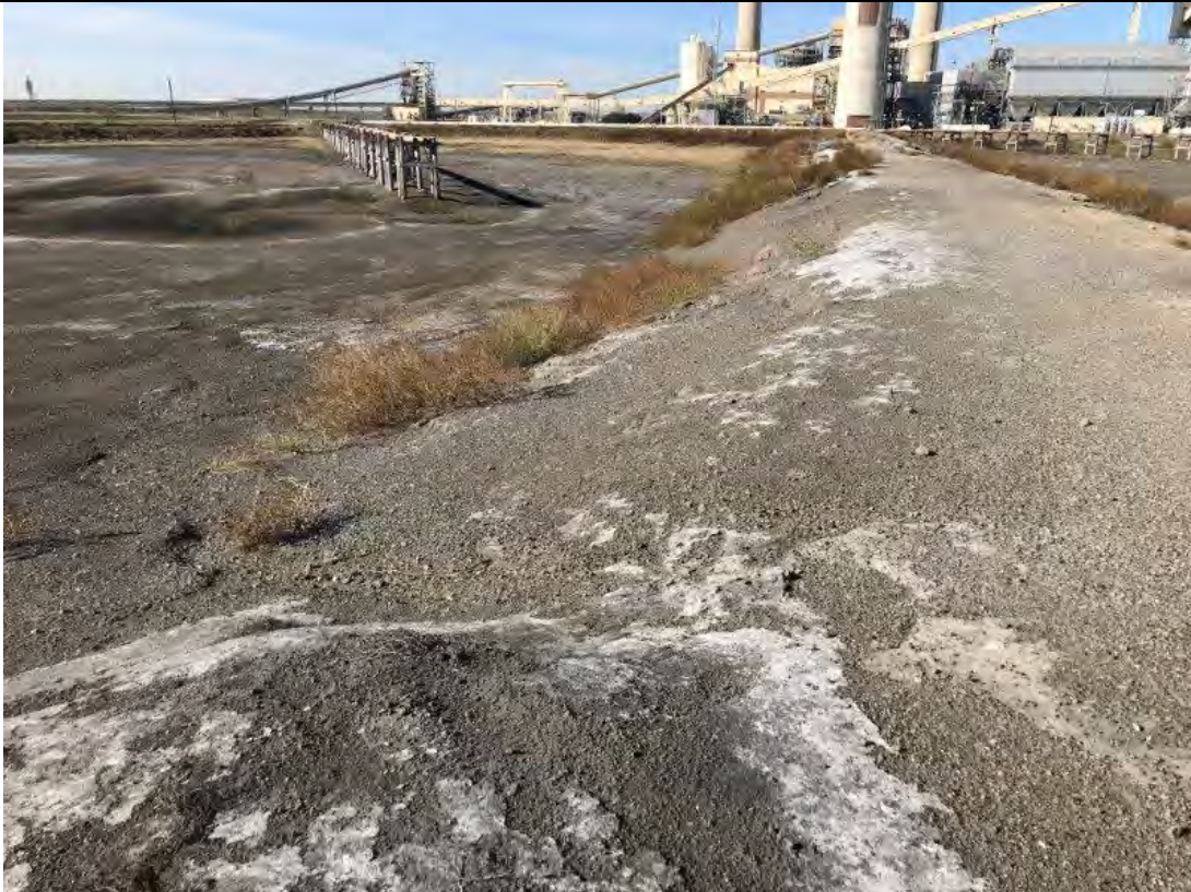
Photograph: 19 South Bottom Ash Pond – standing on northeast corner – facing west. Photo taken 12/19/2019.
