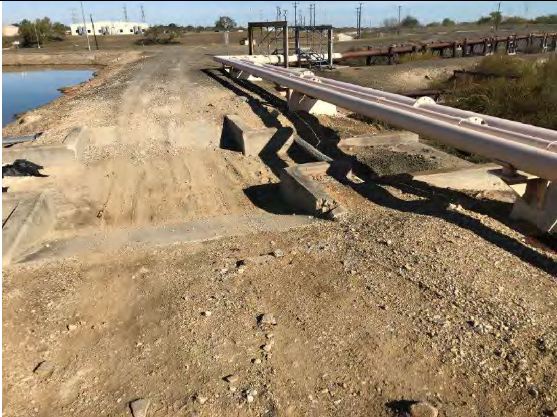
Photograph: 25 North SRH Pond – standing on eastern berm – facing north. Spillway structure. Photo taken 12/19/2019.
