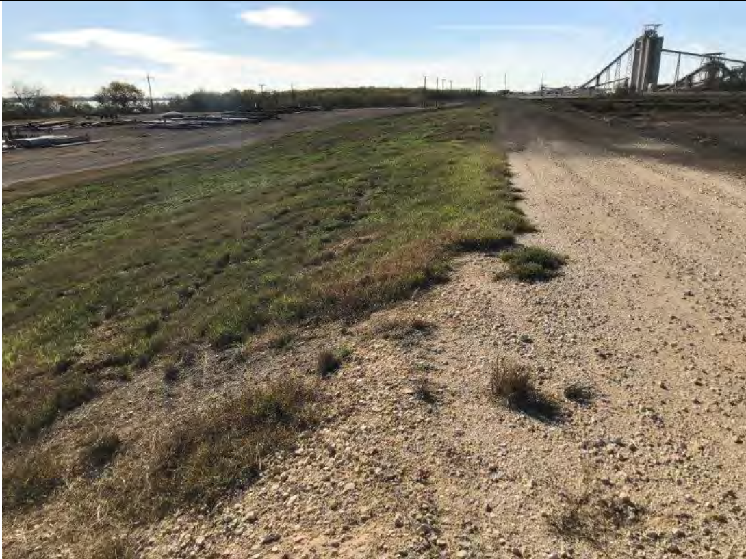
Photograph: 17 North Bottom Ash Pond – standing on northeast corner – facing south. Photo taken 12/19/2019.
