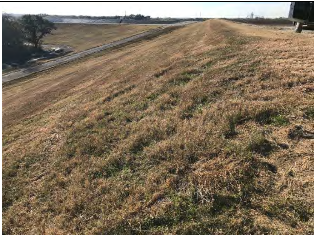
Photograph: 4 Fly Ash Landfill – standing on eastern berm – facing south. Photo taken 12/19/2019.
