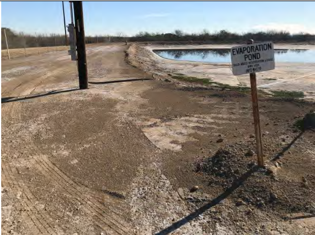
Photograph: 8 Evaporation Pond – standing on the northwest corner – facing east. Photo taken 12/19/2019.
