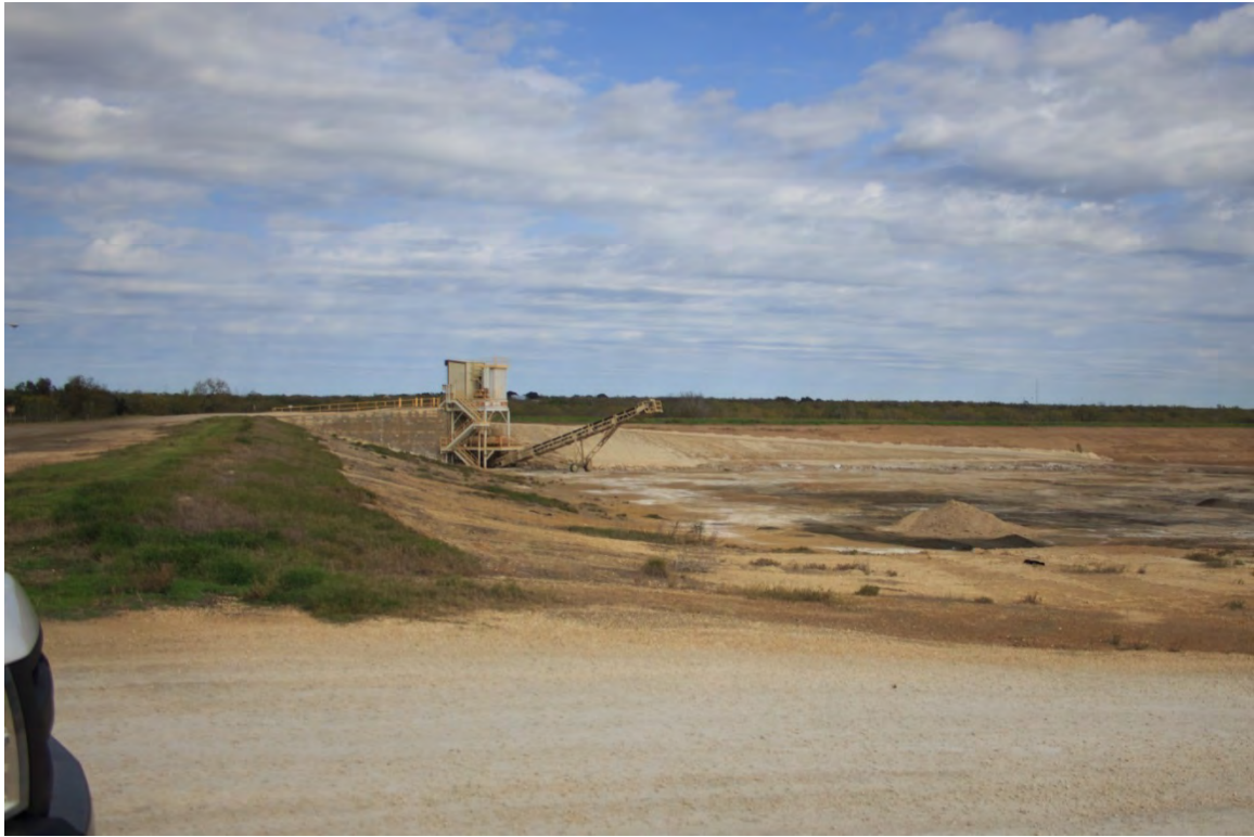
Photograph: 1 Fly Ash Landfill – standing on western berm – facing north. Mobile ash conditioning machine located in northwest corner of landfill. Photo taken 12/16/15.
