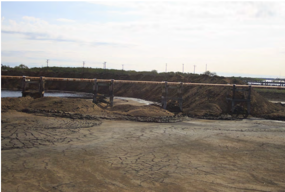
Photograph: 13 North Bottom Ash Pond – standing on western berm – facing southeast. Pond was drained to remove residuals. Photo taken 12/16/15.
