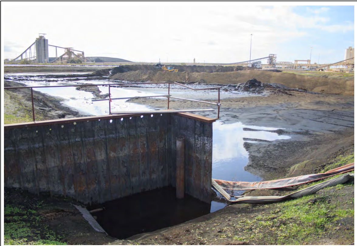
Photograph: 15 North Bottom Ash Pond – standing on northeast corner of pond – facing southwest. Outlet pipe in northeast corner of pond. Photo taken 12/16/15.
