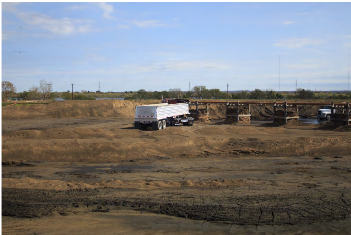
Photograph: 11 North Bottom Ash Pond – standing on western berm – facing northeast. Pond was drained to remove residuals. Photo taken 12/16/15.
