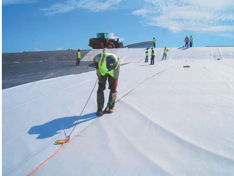
Figure 3-14 Installation of a GCL, showing the geotextile components of the GCL being heat bonded; the black material in the upper left background is 60-mil LLDPE
