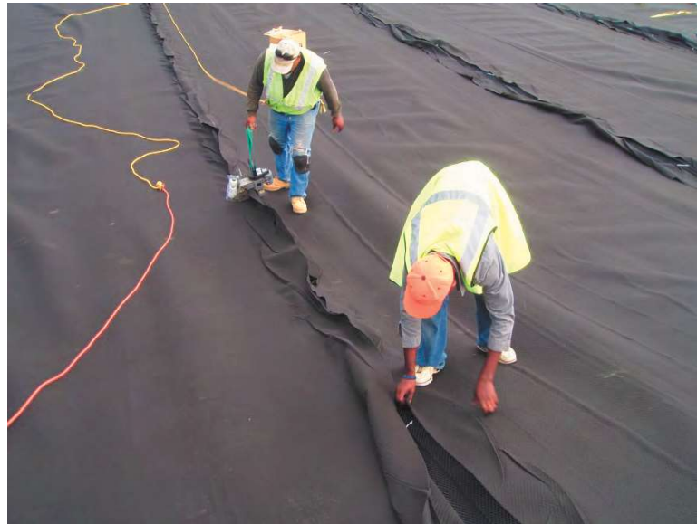
Figure 3-20 Seaming geocomposite panels together using cable ties to secure the geonet and sewing the upper layer of geotextile
