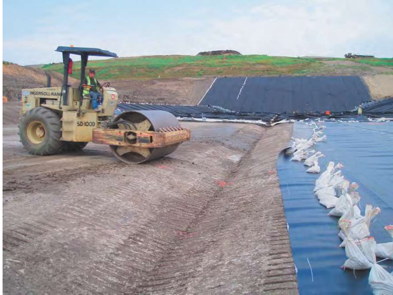
Figure 3-10 Smooth rolling the subgrade prior to deployment of a 60-mil HDPE geomembrane liner
