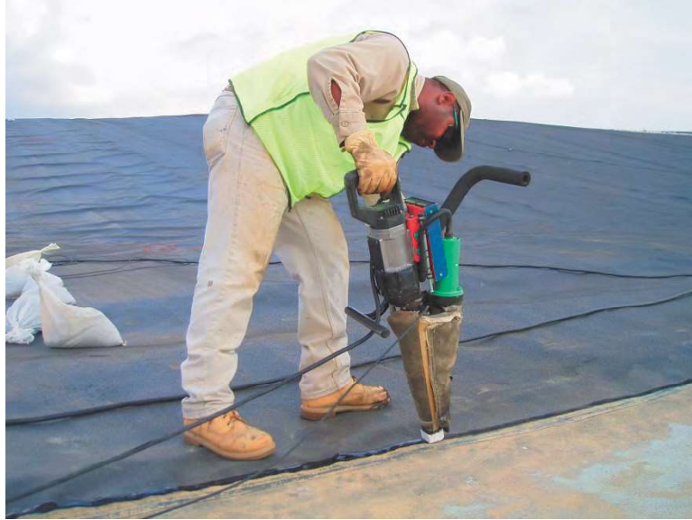
Figure 3-6 Extrusion welding along the tie-in of existing geomembrane to geomembrane in a new construction phase of the landfill
