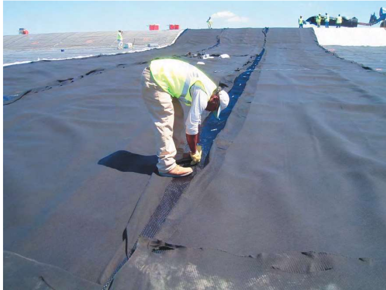
Figure 3-19 Geocomposite installation, showing the geonet overlap being tied together using plastic cable ties
