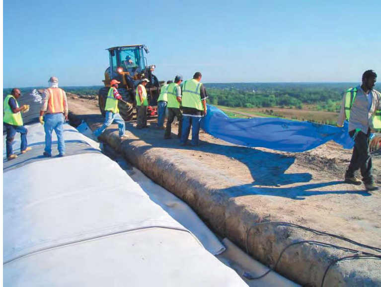
Figure 3-11 Geosynthetics placed in an anchor trench during installation; white material in the foreground is a GCL and dark material in the background is 40-mil LLDPE
