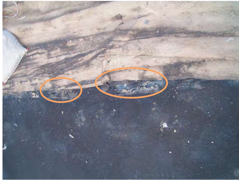
Figure 3-15 Holes burned through geotextile during heat bonding
