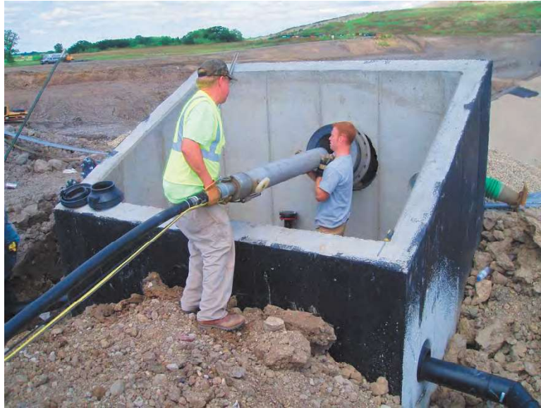
Figure 4-7 Installation of a leachate extraction pump in the sideslope riser pipe through the open riser vault
