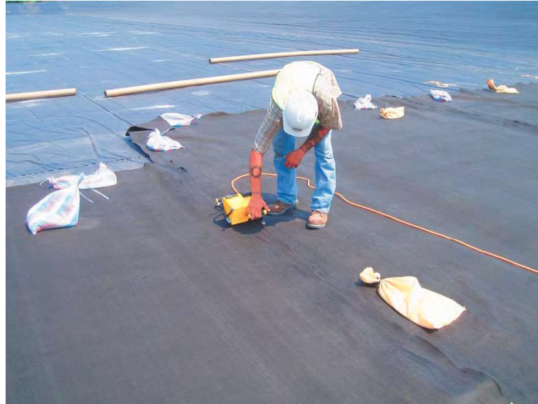
Figure 3-16 Geotextile sheets fusion wedge welded together in the field; the geotextile is being placed over a 40-mil PVC geomembrane, which is visible in the background
