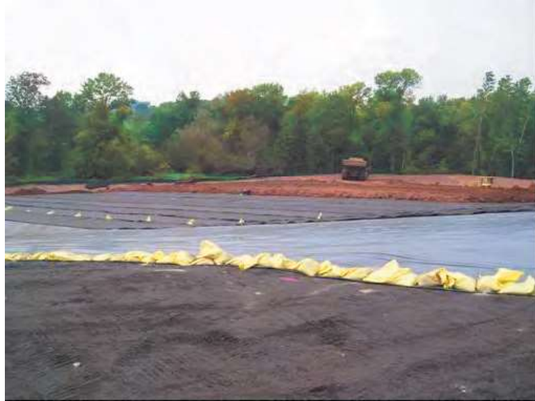
Figure 5-6 Placement of a geocomposite drainage layer (foreground) over a PVC barrier (mid-ground) followed by a soil cover/surface layer (brown material in background)
