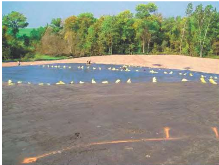
Figure 5-5 Placement of a PVC geomembrane (background) directly over a compacted fly ash subgrade (foreground)
