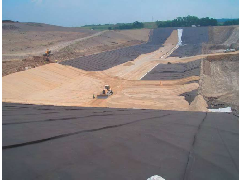
Figure 4-3 Placement of the granular drainage blanket over a 12 oz/yd 2 nonwoven geotextile, which is protecting an underlying 60-mil HDPE Geomembrane
