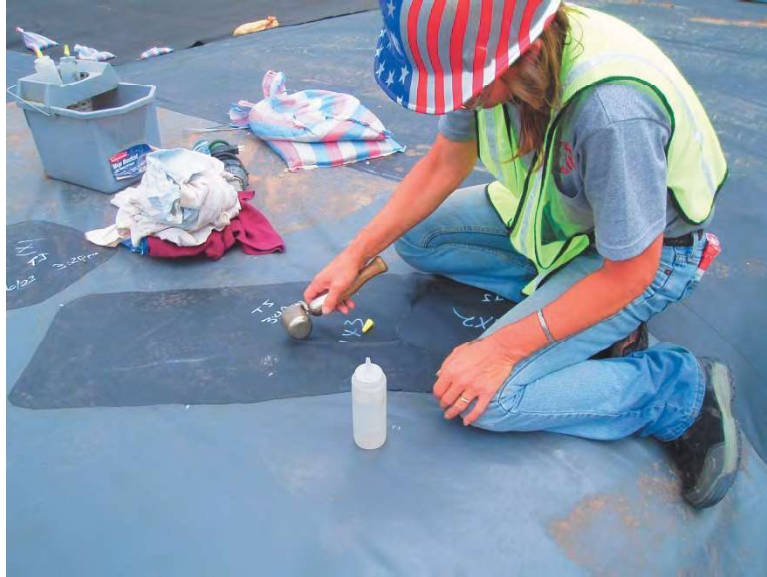
Figure 3-7 Geomembrane repairs performed by solvent welding a patch to the parent PVC geomembrane sheet
