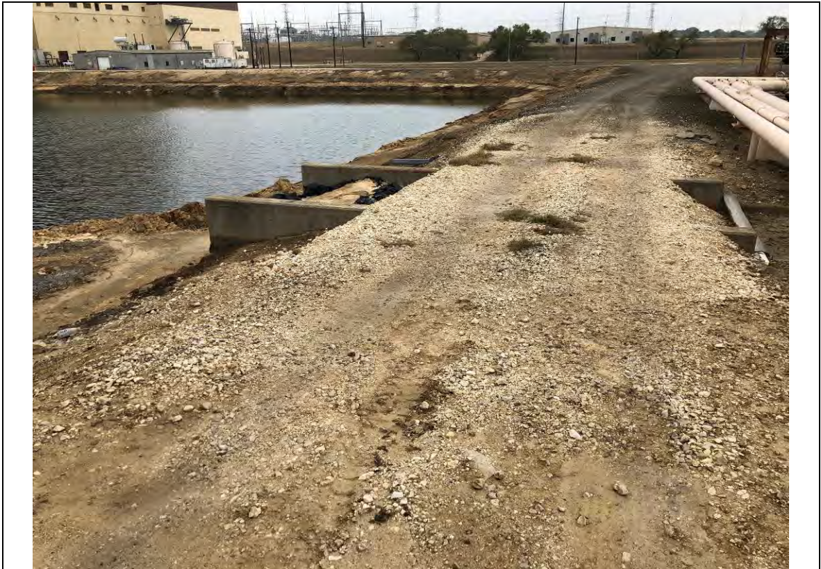
Photograph: 29 North SRH Pond – standing on southeast corner – facing north. Spillway structure. Photo taken 12/15/2020.
