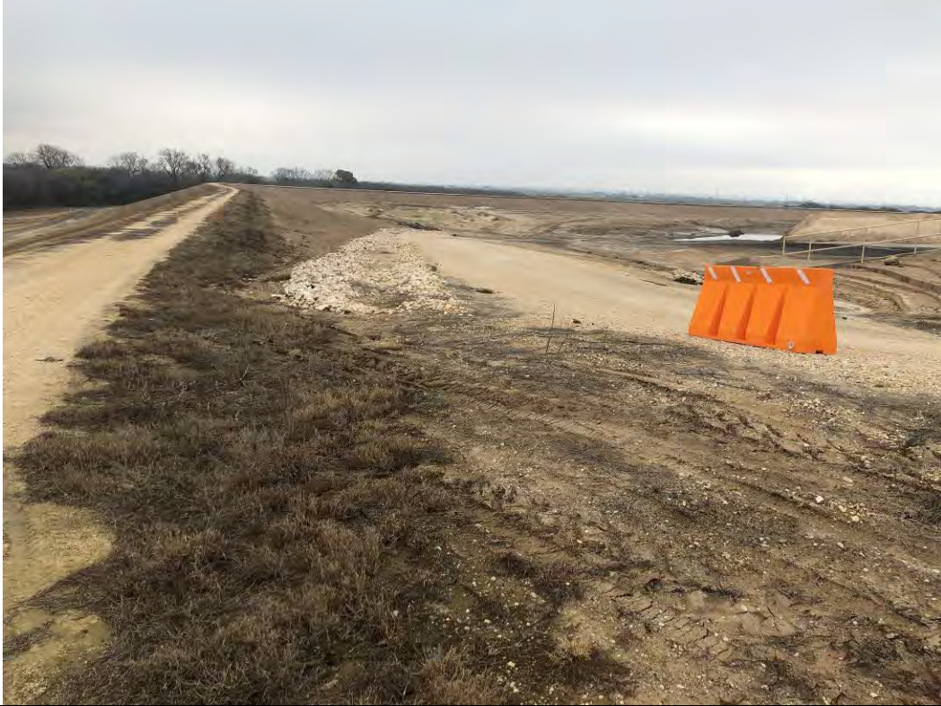
Photograph: 3 Fly Ash Landfill – standing on northwest corner – facing west. Photo taken 12/15/2020.
