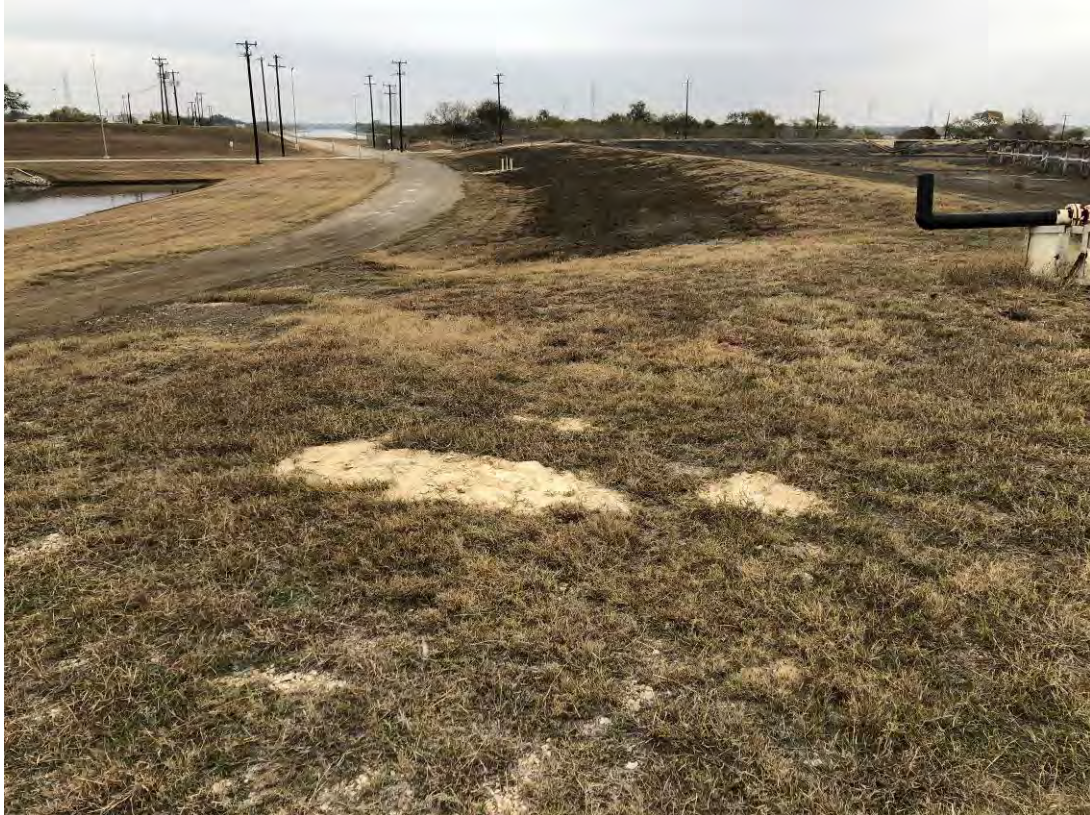
Photograph: 19 North Bottom Ash Pond – standing on southwest corner – facing northeast. Photo taken 12/15/2020.
